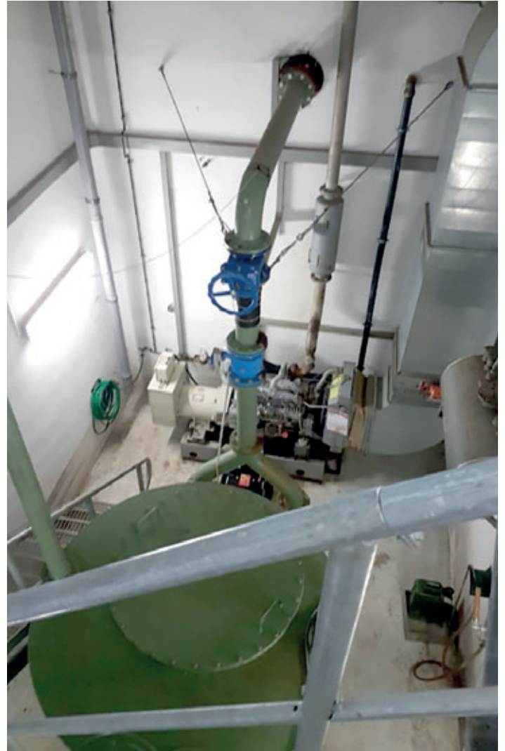
Blick in das Pumpwerk
